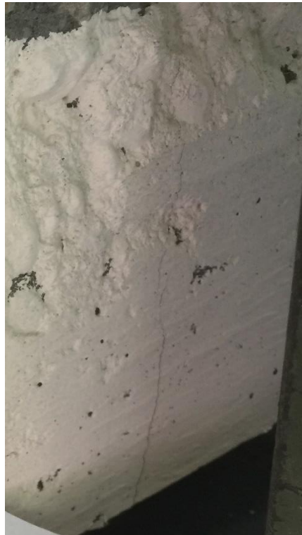
Figure 4-2 First Crack in Specimen 1
